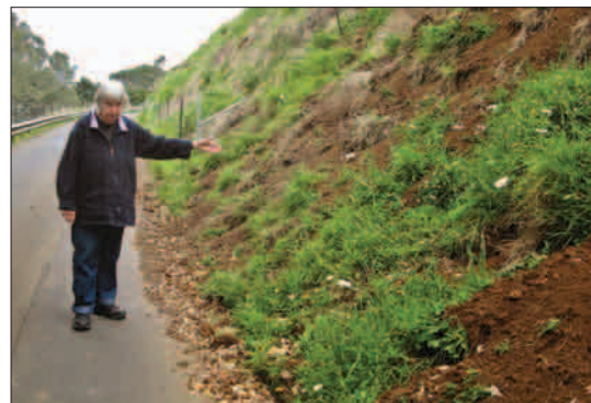
Sue Bulmer examines erosion in the historic reserve. A failed pātītī trial area is visible on the bank behind her.
