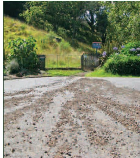
Poor drains and lack of maintenance caused this 2007 washout after heavy rain. FoM volunteers have built water bars and halted much of the track flooding and erosion.
